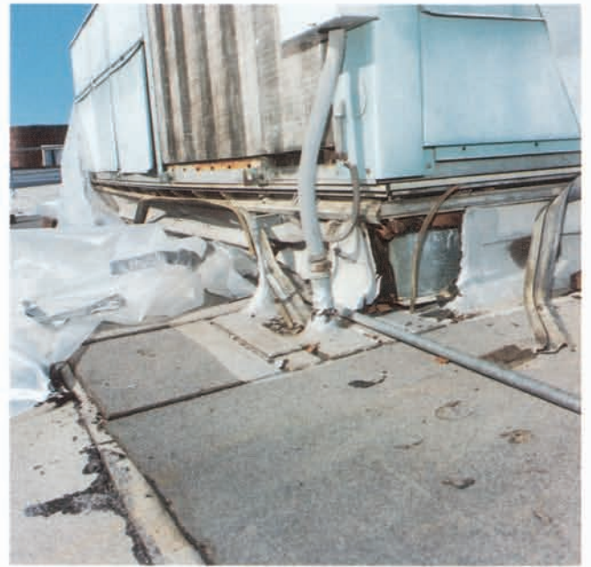
Figure 16. Isolated aluminum roof curbs failed because of the lack of structural strength of the aluminum sections (roof location, 4 stories, approximate maximum seismic excitation - 0.3 g horizontal, 0.22 g vertical).
