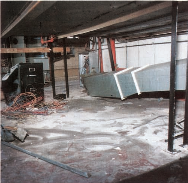
Figure 12. Duct failure resulted when sway braces were omitted (4th floor location, 4 stories, approximate maximum seismic excitation - 0.4 g horizontal, 0.28 g vertical).
