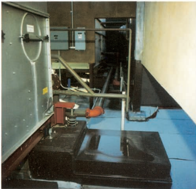
Figure 7. The cooling tower is mounted on a proper structural frame with all-directional Z-1011 seismic snubbers. The result is no failure with the cooling tower remaining operational (roof location, 8 stories, approximate maximum seismic excitation - 0.45 g horizontal, 0.32 g vertical).
