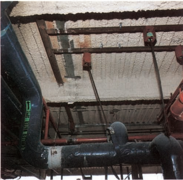
Figure 11. Pipe support rods were displaced which caused the piping to distort. The pipe distortion is expensive to repair (8th floor location, 8 stories, approximate maximum seismic excitation - 0.36 g horizontal, 0.22 g vertical).
