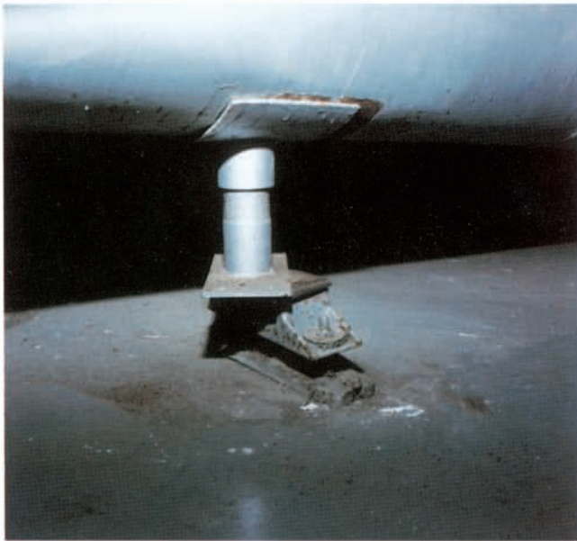
Figure 6. The attachment of the stand to the pipe and to the top of the machinery mount is not proper. This allowed the stand to shift off the mounting (basement location, 6 stories, approximate seismic excitation - 0.3 g horizontal, 0.25 g vertical).
