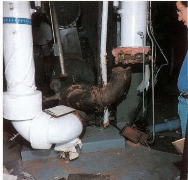
Figure 14. Piping failures at interface connections can be prevented with the use of elastomeric joints (15th floor location, 15 stories, approximate maximum seismic excitation - 0.4 g horizontal, 0.28 g vertical).
