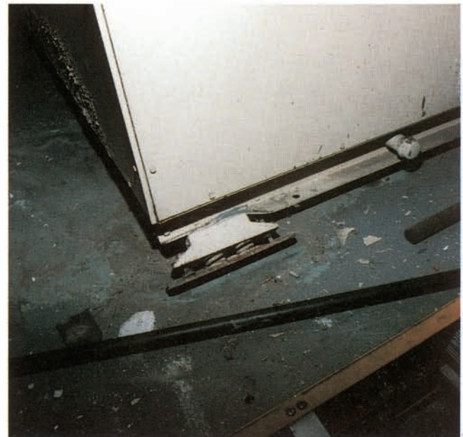
Figure 5. Direct mounting of vibration isolators can result in failure if the machinery frame is not adequate and local buckling occurs (roof location, 2 stories, approximate maximum seismic excitation - 0.42 g horizontal, 0.3 g vertical).
