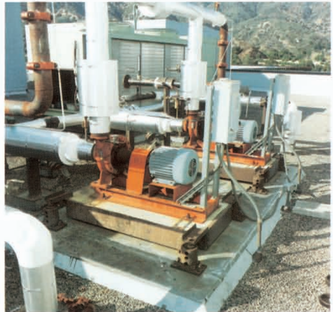
Figure 8. The seismic snubbers are built into the vibration isolators. The system was properly adjusted and withstood the effects of over 2 g input and remained operational. The mounting type is Mason SSLFH (roof location, 7 stories, approximate maximum seismic excitation - 2.3 g horizontal, vertical n/a).
